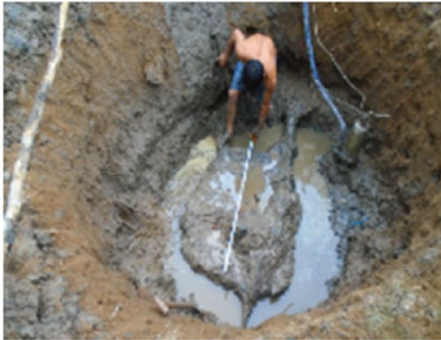
(a) The top of the pilot column appeared at a depth of 1.5 m
