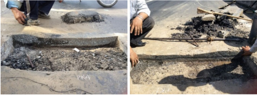
Fig. 1 Typical rutting profile of flexible pavements in Vietnam. Photos taken by BMT J.S.C. in May 2014 at National Highway 1A, located between An Suong and An Lac intersections
