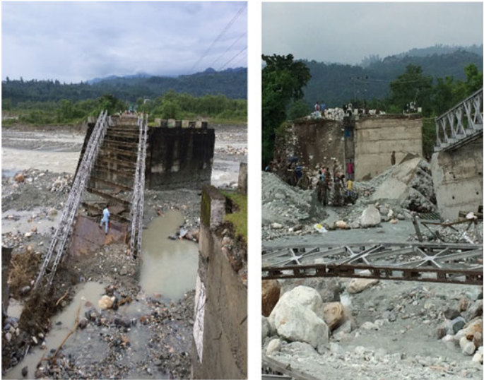
Fig. 2 Fallen bridge due to scouring
