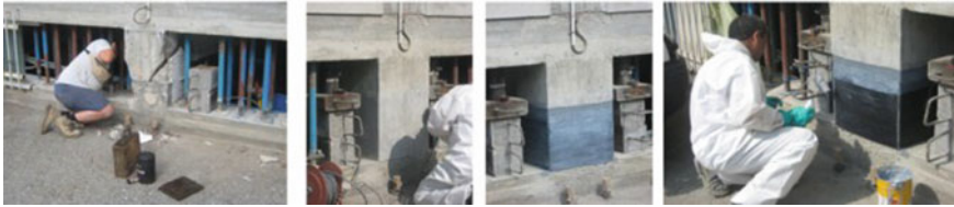
Fig. 6 Illustration of steps for reinforcing reinforced concrete columns with basalt-BFRP fiber reinforced material
